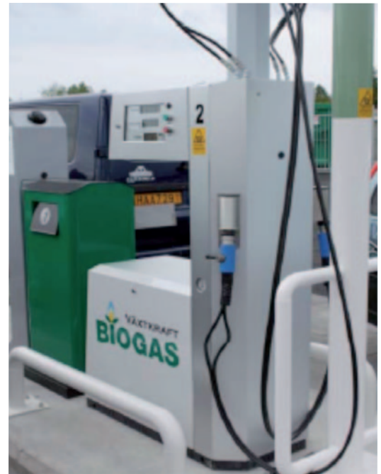
Project MADEGASCAR Malardalen Energy Agency. Gas filling station (Västerås).
