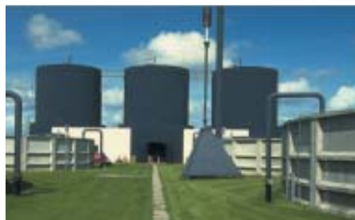
Large Scale Centralised Co-digestion Plant Lemvik, Denmark (Picture courtesy of Teodorita Al Seadi, Denmark)
