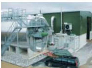
Kompostgas plant in Oetwil, Switzerland
