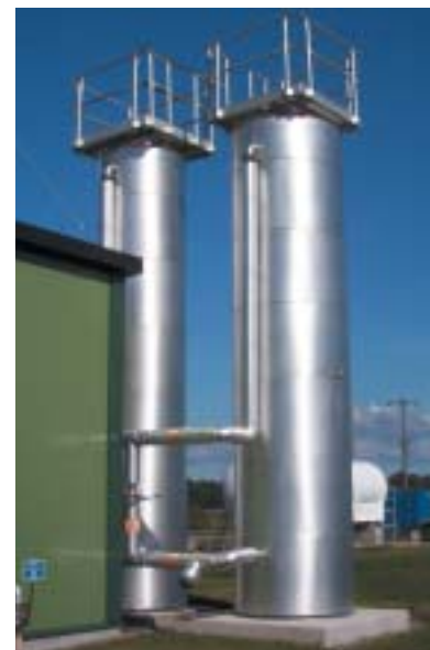
Vessels containing iron oxide that removes \text{H}_2\text{S} from the biogas
