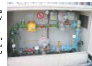
Gas injection into the natural gas grid in Samstagern, Switzerland
