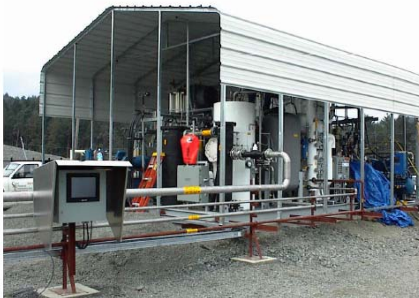
Figure 3-7 Skid-mounted 225-gpd landfill gas liquefaction Hartland Unit, located in Victoria, B.C. developed by CryoFuels Systems, Inc. (source: CryoFuels Systems, undated)
