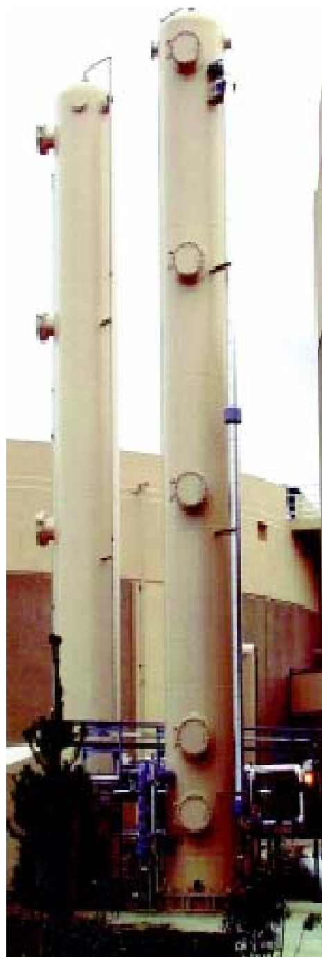
Figure 3-1 Carbon dioxide absorption towers at the King County South Wastewater Treatment Plant
